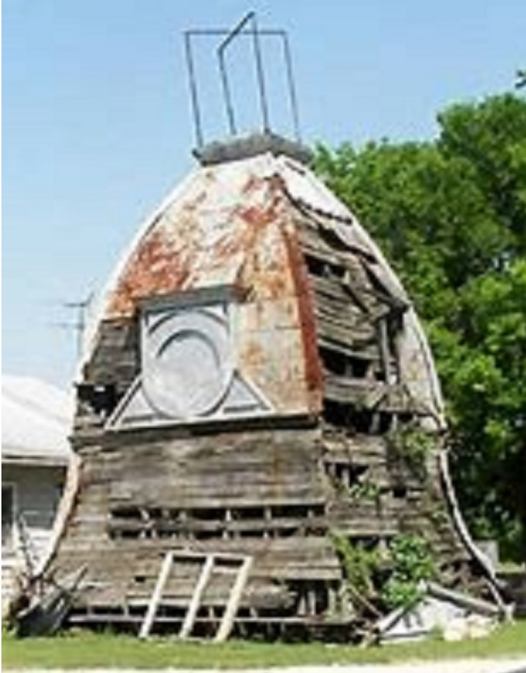
THE ORIGINAL BELL TOWER BEYOND REPAIR
